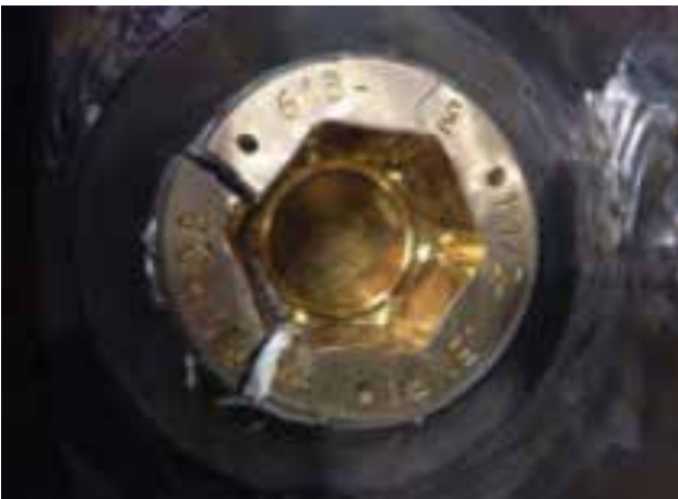
Figure 2: Example of a cracked socket caused by a tool which was not aligned in the axis of the socket during installation
